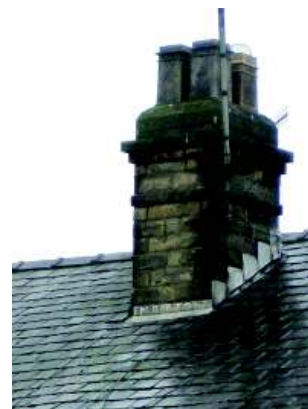
Picture 28 Chimney stack on Bingswood Avenue
